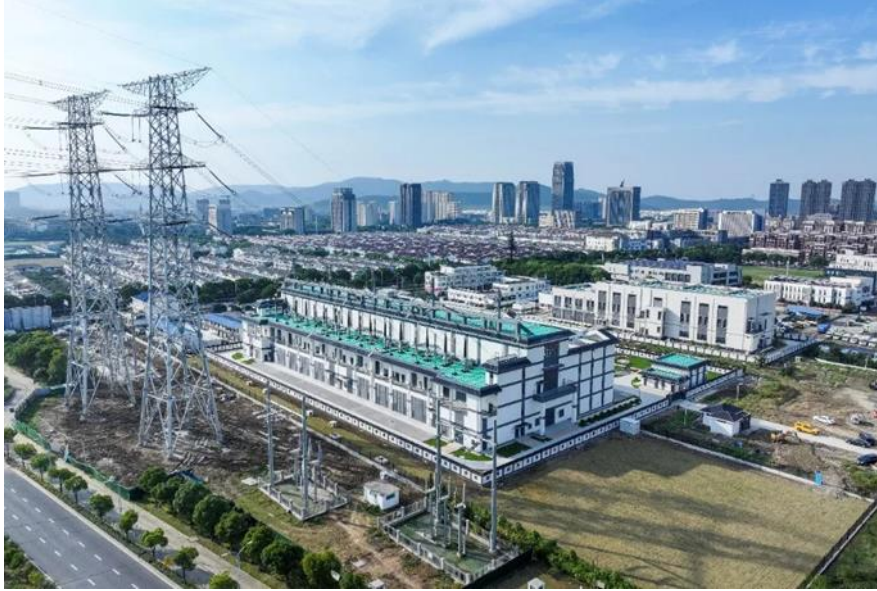
Fig. 3. 500 kV Transmission substation in suburban Nanjing, Jiangsu Province, China– study site for hazard monitoring
