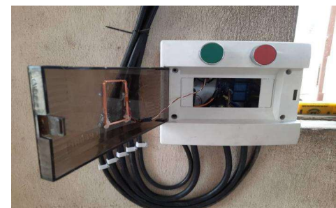
Fig. 16. The control system module
