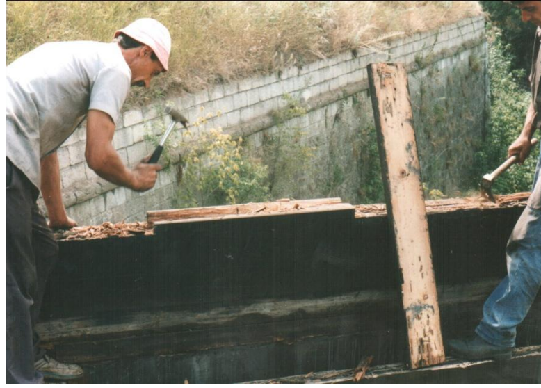
Figure 1. Deterioration of the main beam of the timber bridge
